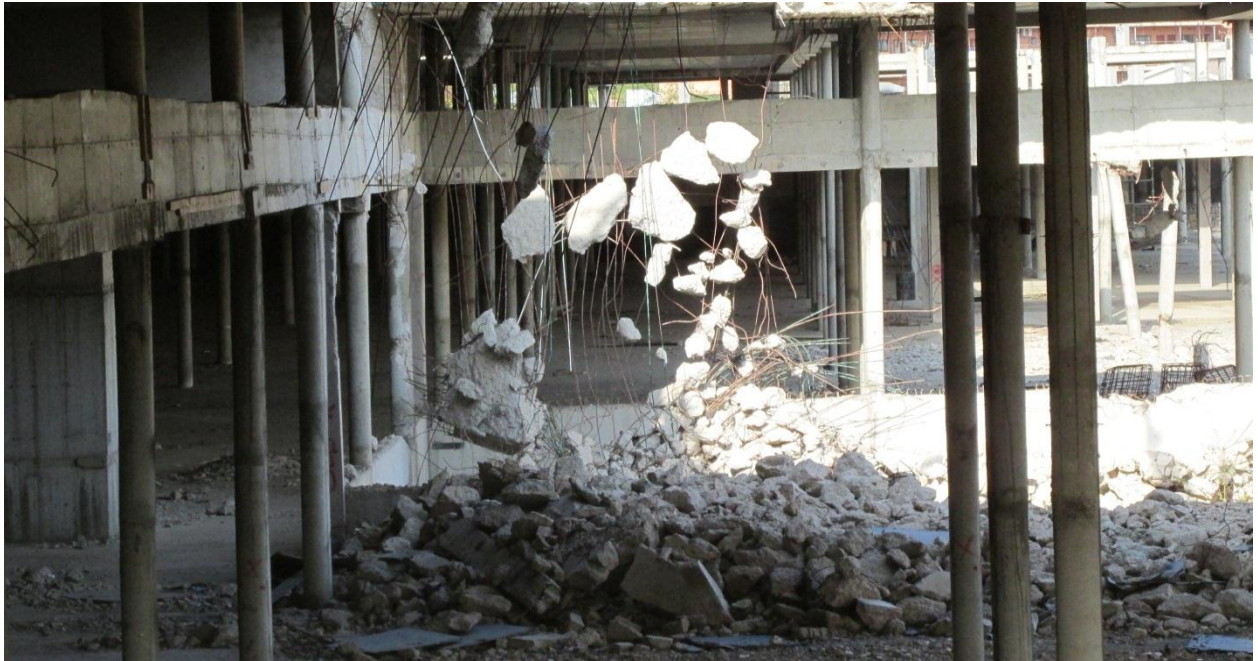
Figure 4.11: Extent of the Tongaat mall collapse – slab view (Source: Van Eeden, 2015)
