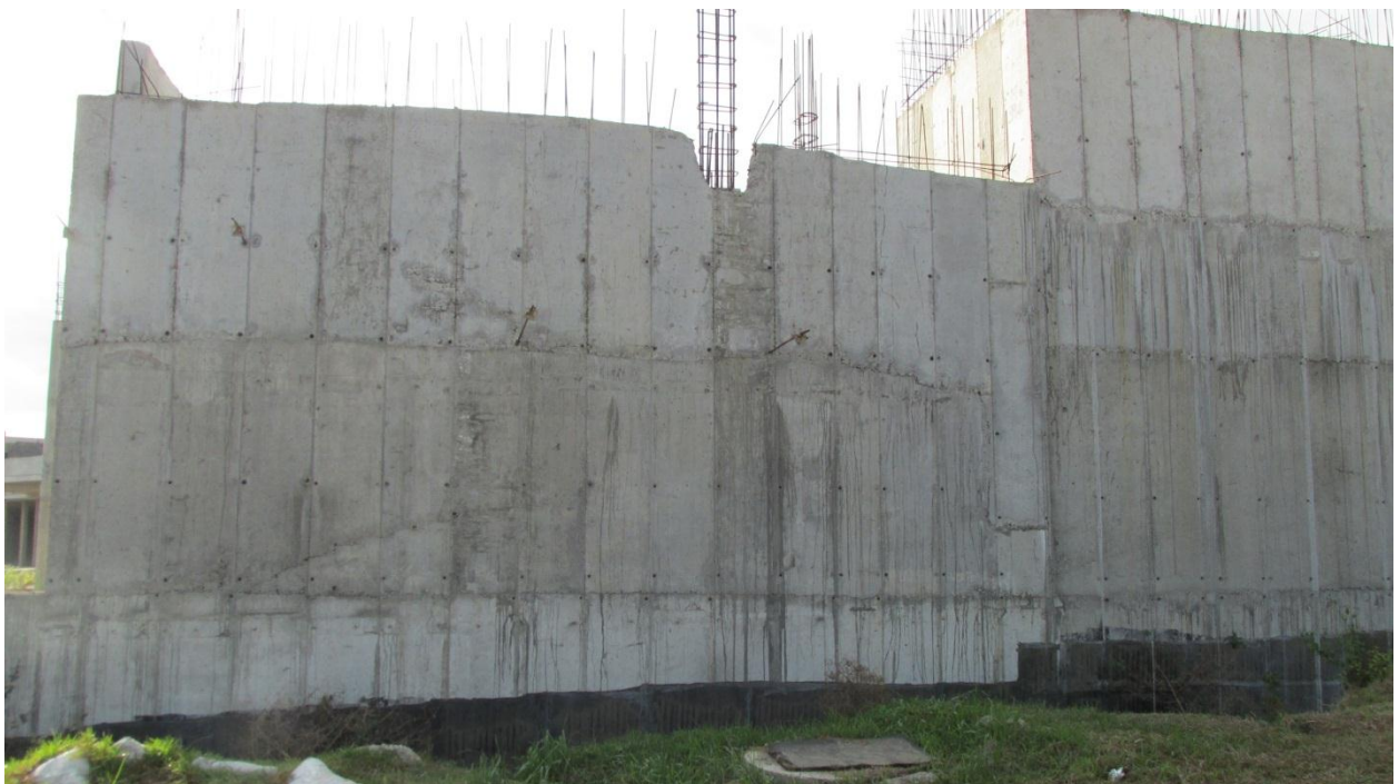
Figure 4.14: Example of poor concrete work evident in Tongaat mall (Source: Van Eeden, 2015)
