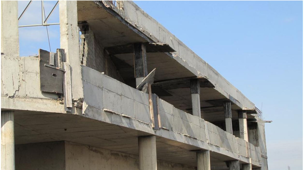
Figure 4.13: Example of poor construction found in the Tongaat mall (Source: Van Eeden, 2015)
