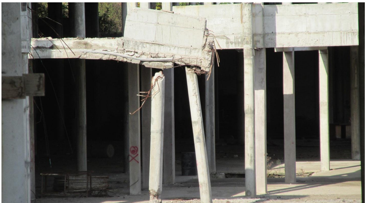
Figure 4.6: Collapsed slab and dismembered columns (Source: Van Eeden, 2015)
