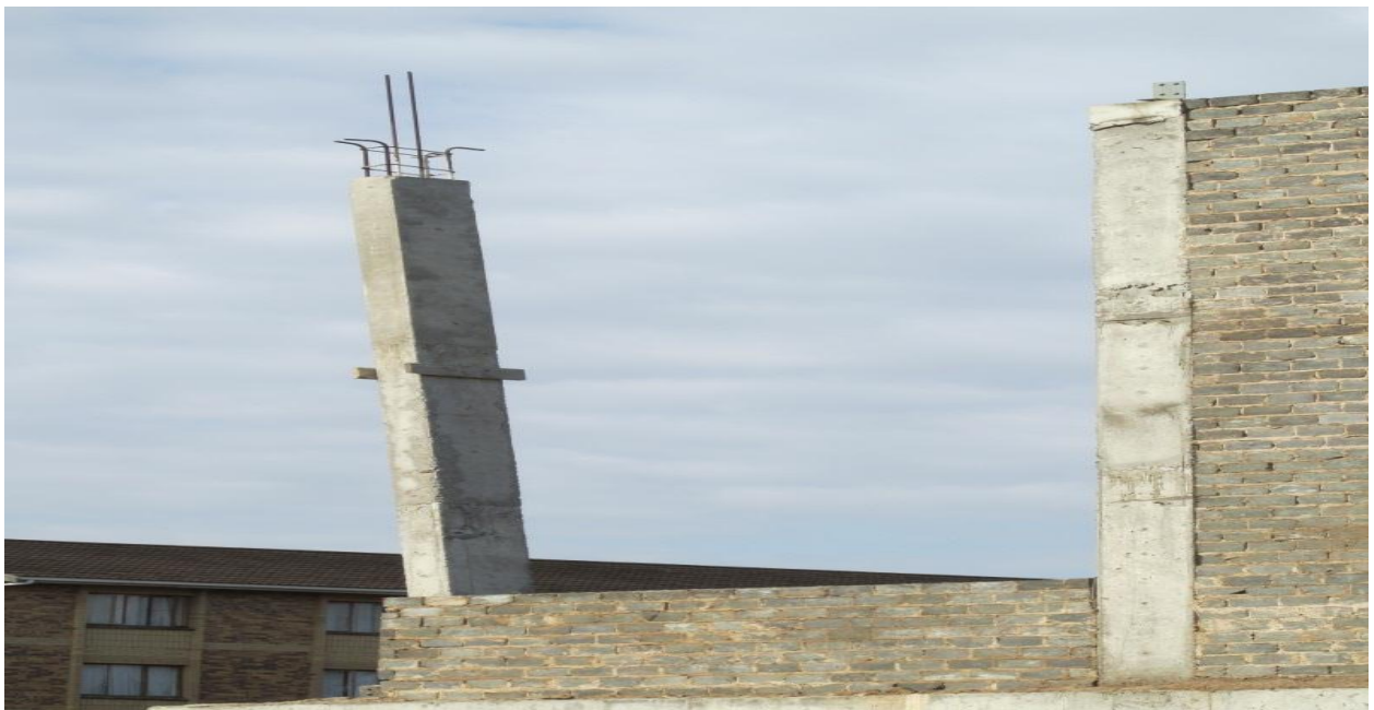
Figure 4.8: Deflection of columns that was notable throughout the site (Source: Van Eeden, 2015)
