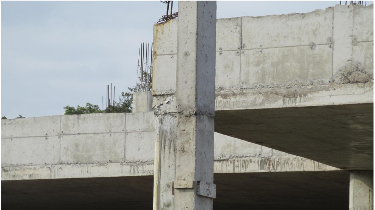
Figure 4.7: Shoddy construction work in terms of column construction that was notable throughout the site (Source: Van Eeden, 2015)
