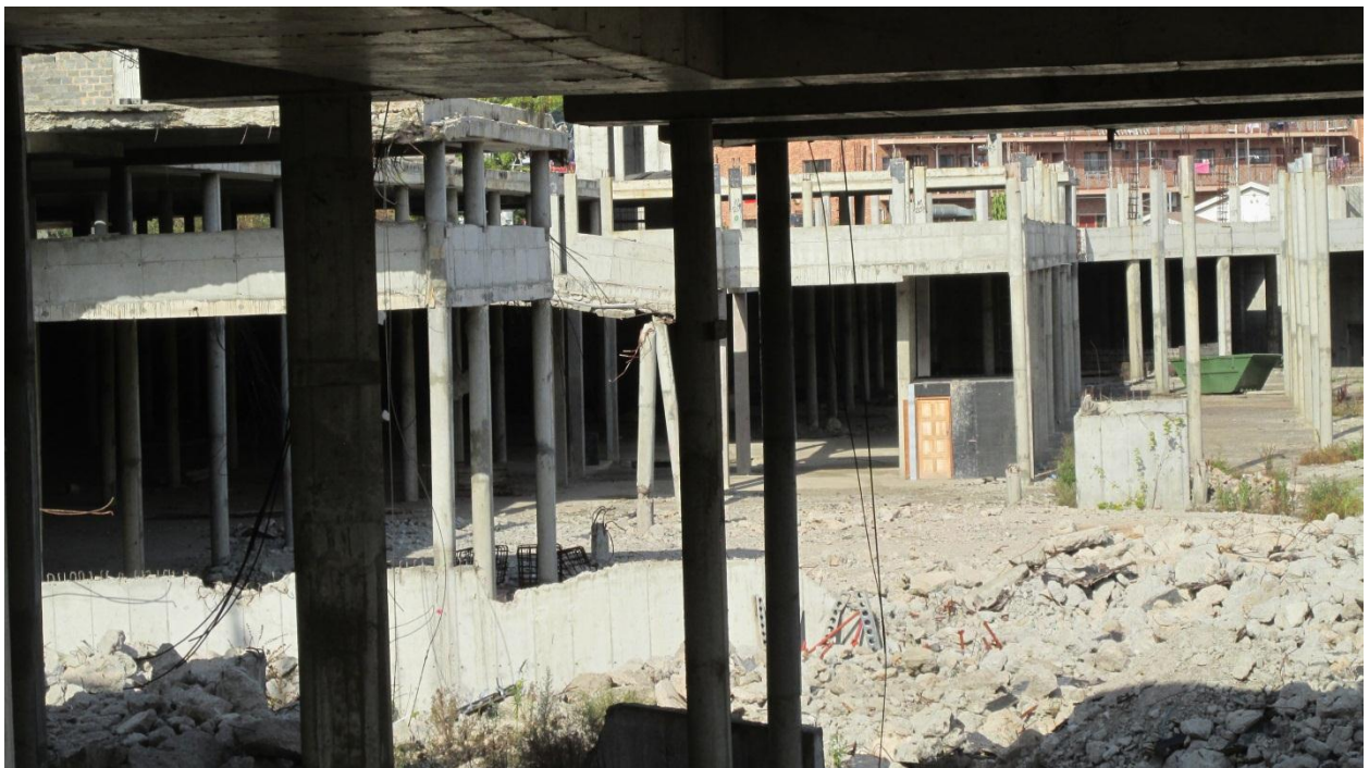
Figure 4.12: Extent of the Tongaat mall collapse – centre view (Source: Van Eeden, 2015)
